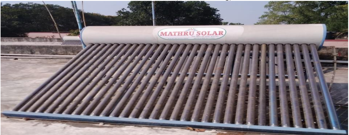
Solar Water Heaters in Kaveri Ladies Hostel, Karnatak Science College, Dharwad.
