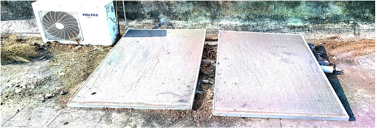
2 KVA Solar Power Generation Unit in IQAC Office (Office Building)
